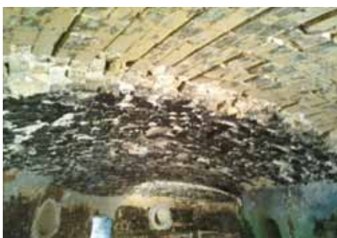
Fig. 5 Condition of lining with semi-silica bricks two years after capital repair
