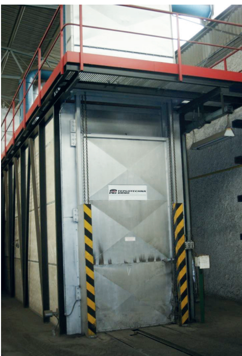
Fig. 1 Exit of the tempering kiln
