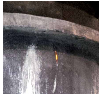
Fig. 1 Example of a vertical crack below the top stiffener band
