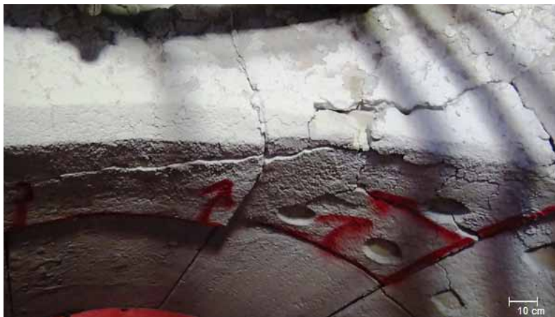
Fig. 15 Front view of the lining failure and crack propagation found in a bullnose area with ceramic anchors in Region 1
